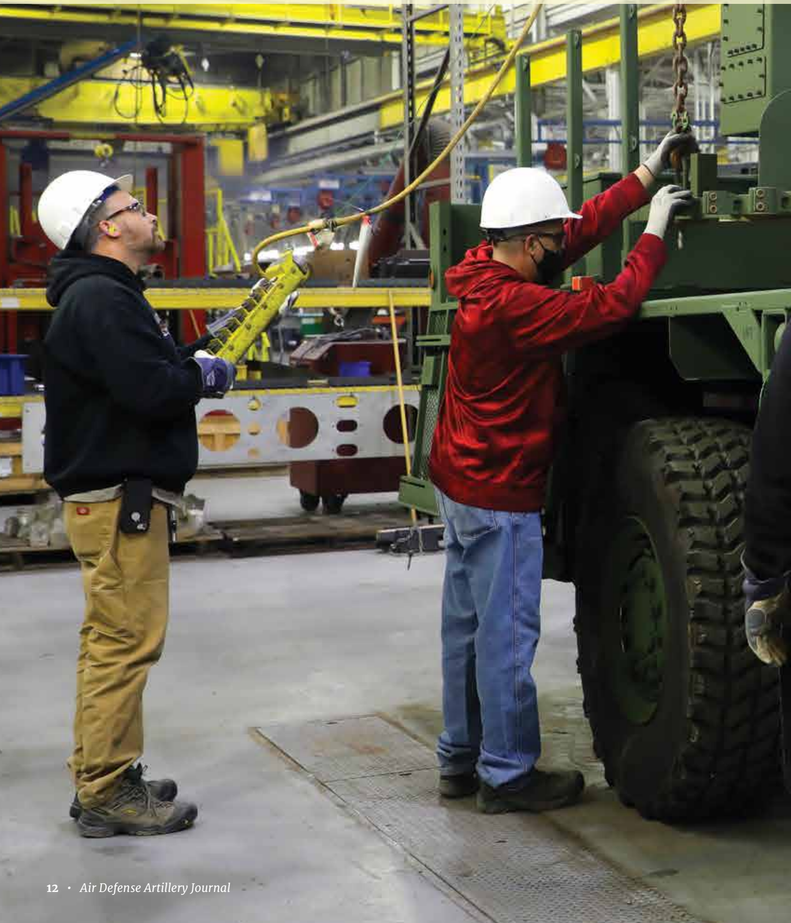
Mike Piper, ordinance equipment mechanic, Chad Elliott, heavy mobile mechanic contractor, and Jared Mayhugh, heavy mobile mechanic contractor, mount a new-build A3 Sentinel radar onto a M1082 LMTV trailer at Letterkenny Army Depot March 3, 2021. (U.S. Army photo by Pam Goodhart)
