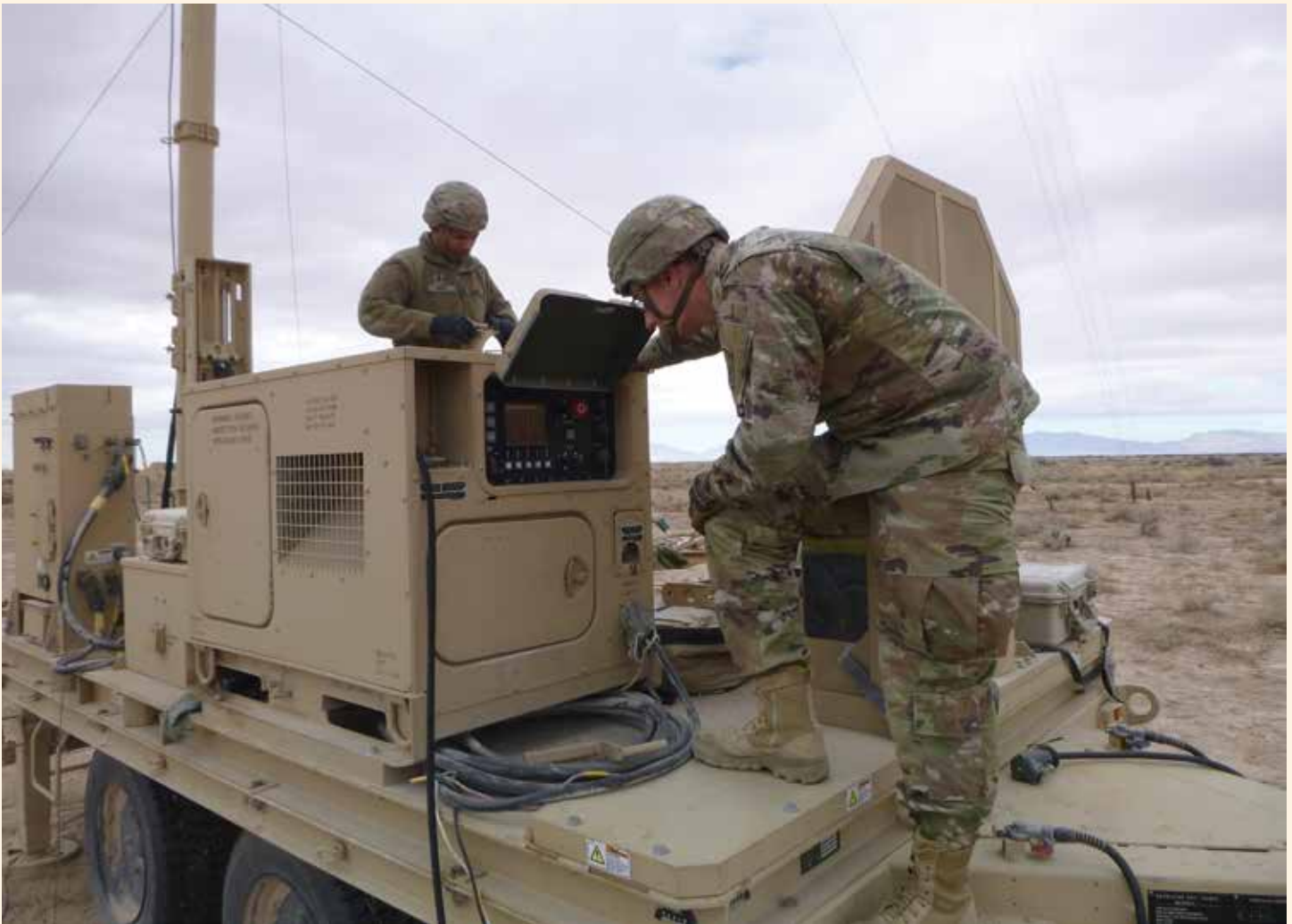
SPC Norman Parks (left), and PFC Jonathan Oliver, Engagement Operations Center crewmembers with 3rd Battalion, 43rd Air Defense Artillery Regiment, perform preventative maintenance checks and services (PMCS) on a generator. Parks reads the PMCS steps out loud so Oliver can perform a fault isolation on the AIAMD IFCN Relay. (Photo by SSG Christopher Pabst, Air and Missile Defense Test Directorate)
