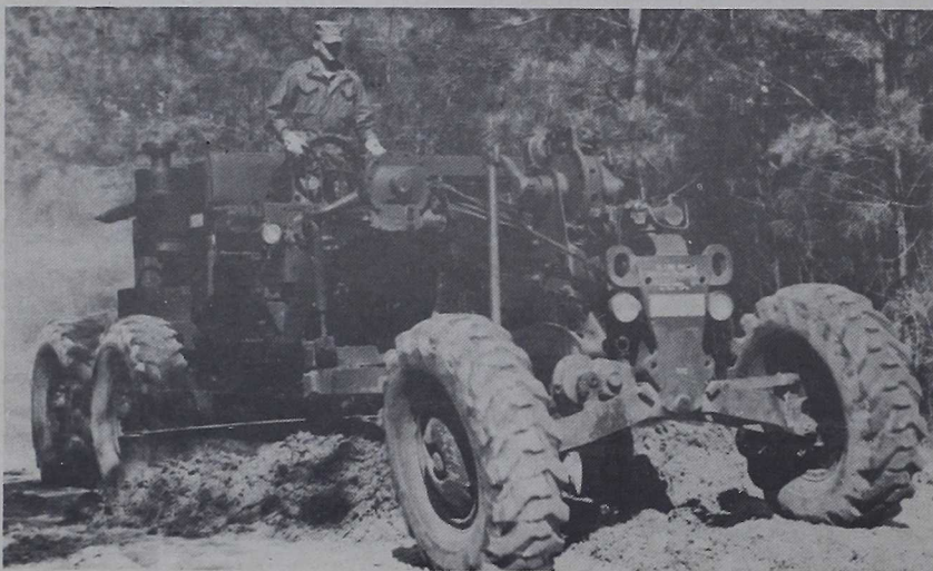
GRADING THE ROAD — A road grader from 8th Engineer Bn. makes quick repair work on a forest road.
