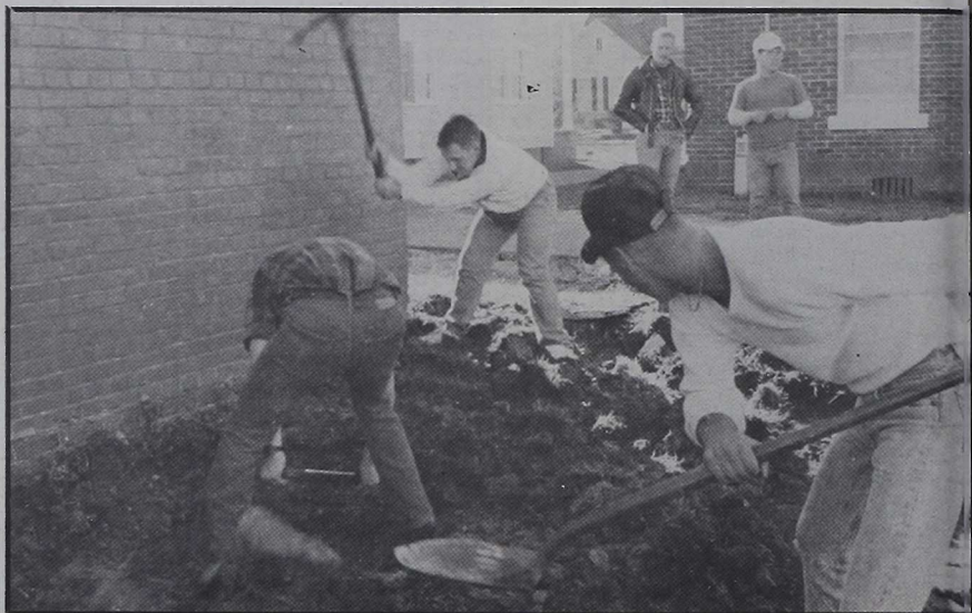
When artillery goes to the field, Marines do a lot of digging. At the Jacksonville shelter for battered women and children, they turned their picks and shovels to create a cement slab for a garbage dumpster.
