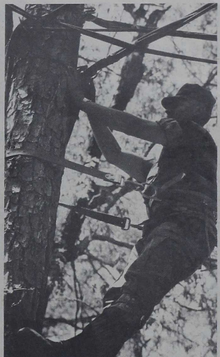
Private First Class Kevin D. Francis, wireman, installs telephone lines on tree trunks.
