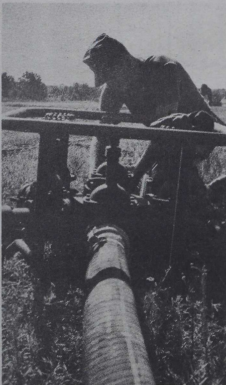
Lance Corporal Richard Ellis, 1st Bulk Fuel Company, connects a dispenser hose to a spider manifold on a tank farm.
