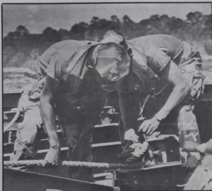
SECURING THE LINES — Basic engineer students work to secure lines from one of the boats to the bridge.
