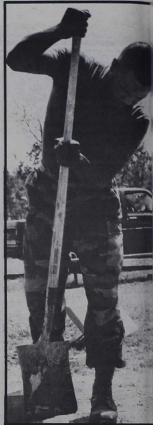
SPECIAL SERVICES—(Above) Cpl. M.G. Williams, Consolidated Special Services, MCB, digs a hole to place the foundation for first base. GRATING—(Left) Lance Cpl. T. L. Steedley, grounds and maintenance, Consolidated Special Services, smooths out the dirt of the women's softball field at French Creek.
