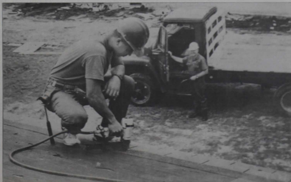
BUC apprentice John Nogueras nails on roof shingles as part of the renovation of the buildings.
