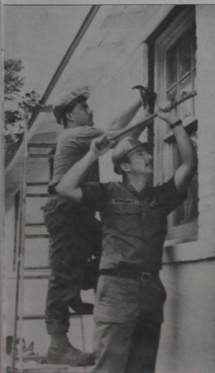
T2 Timothy McIntyre, left, and SW1 John Lyberanec install new windows in one of the OTG buildings.
