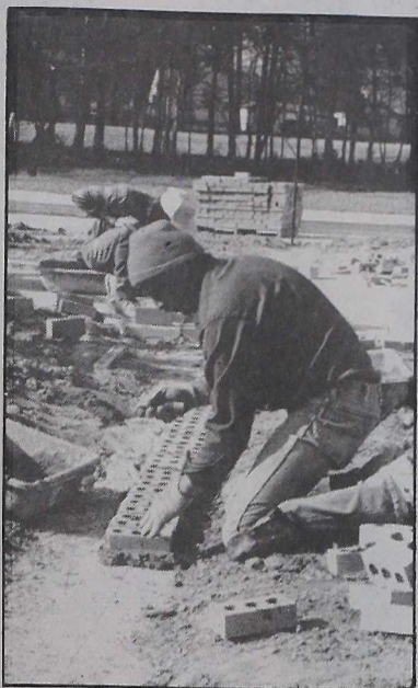
Contractors put finishing touches on what is now the North Carolina Veteran's Cemetery.
