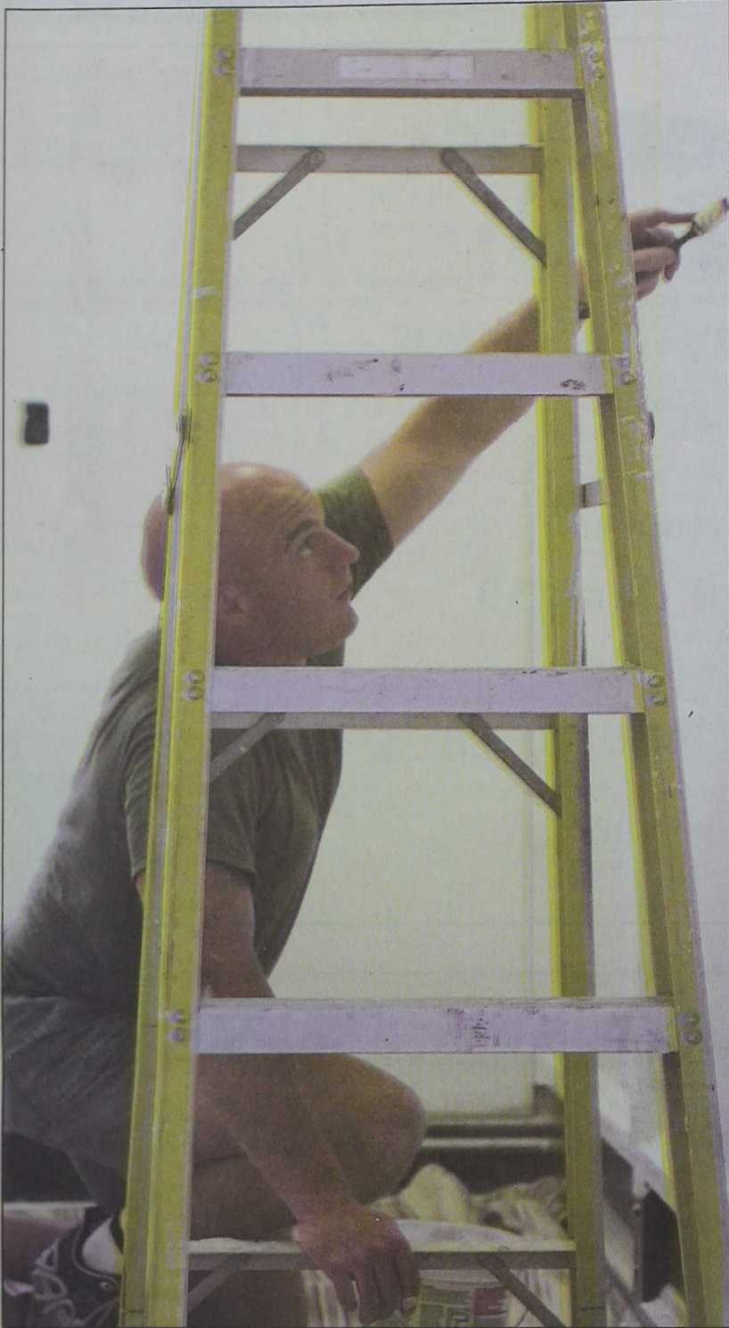
Sgt. Lafferty adds a coat of paint to the newly remodeled RSU barracks. The building houses the various units who come aboard to conduct training.
