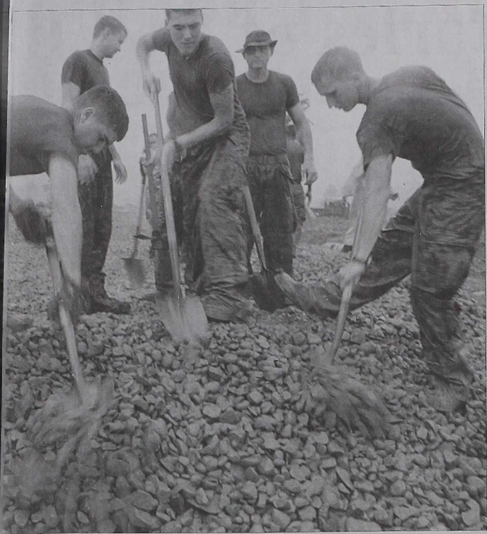
Cpl. Martin R. Harris Leyte, Philippines: Marines with combat engineers detachment, 31st Marine Expeditionary Unit, shovel gravel to level off a hill on the road they are building to the landslide disaster area in Southern Leyte, Philippines.
