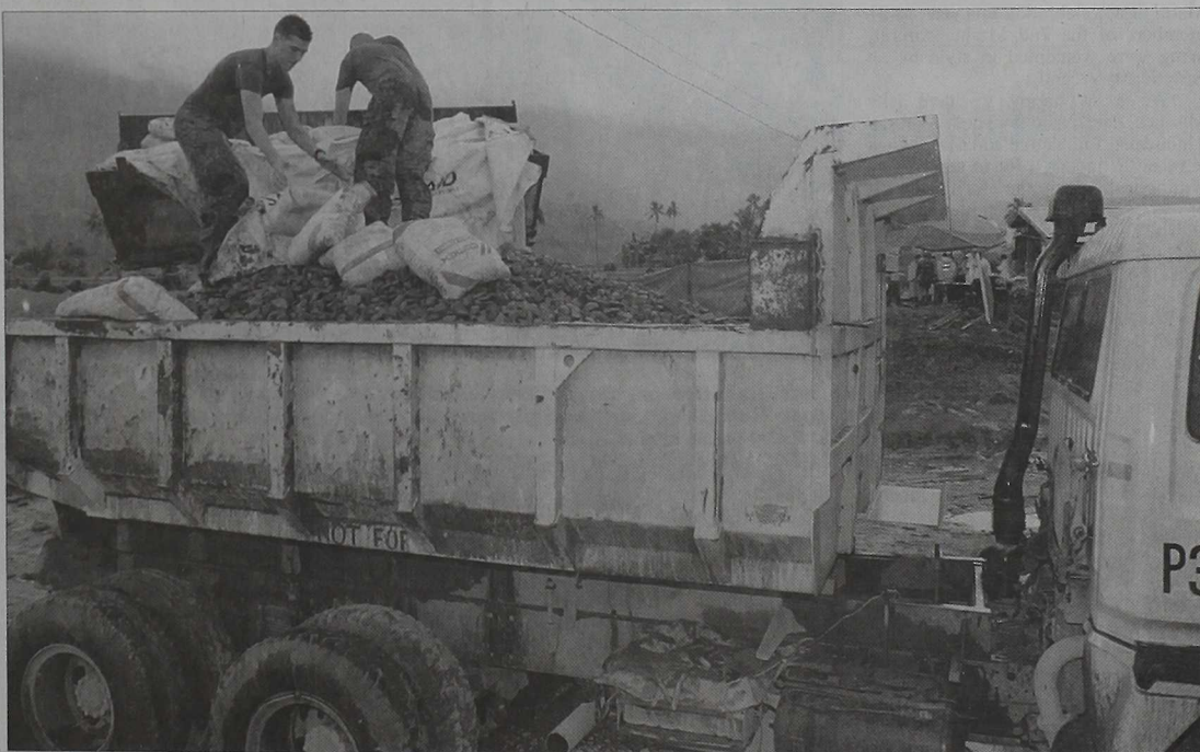
Cpl. Martin R. Harris Southern Leyte, Philippines: Marines with combat engineers detachment, 31st Marine Expeditionary Unit, are mixing bags of concrete to help the gravel mess with the logs.
