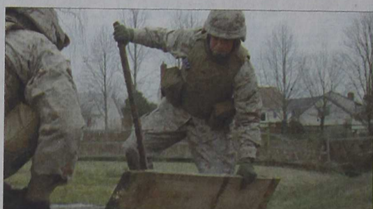
Virginia Beach, Va.: Cpl. Kaleb P. Griffel, 24th MEU, rips wood planks from a foot bridge being demolished at Salem Woods Residential Park.
