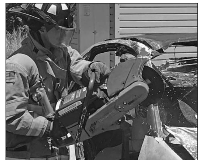
Pine Bluff Arsenal firefighter Michael Harrington using the K12 saw to cut the “A” Post during training held in July. The training is part of the firefighter’s required training. Crews discussed and exercised four essential steps to a vehicle accident: Scene size up; vehicle stabilization; patient extrication and patient care. U.S. ARMY PHOTOS BY DES
