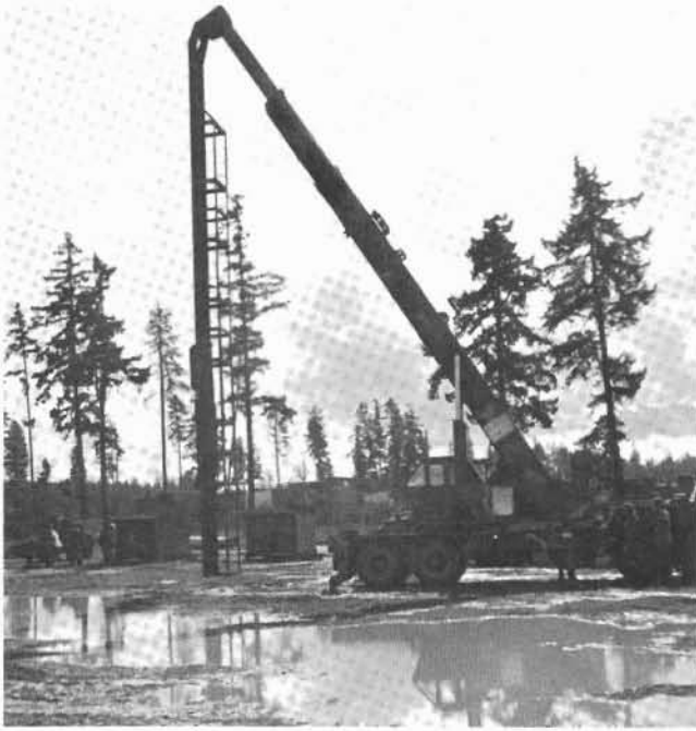
Lifting and loading specialists, MOS 62F, drove piles and used cranes and forklifts during the battalion FTX. (Photos by Robert J. Walz.)
