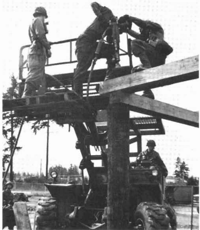
General construction machine operators, MOS 62J, pinned timbers to piles and provided lighting to various project sites.
