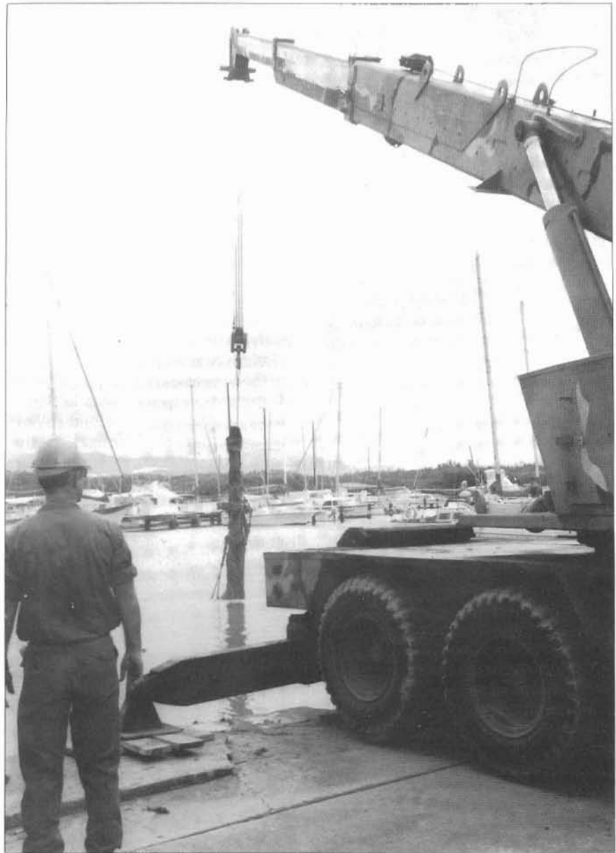
Decaying marina pier-poles being removed at low tide. Working from a barge, A Co. put in 70 new piles in 15 days—five times more than the Navy thought possible.
