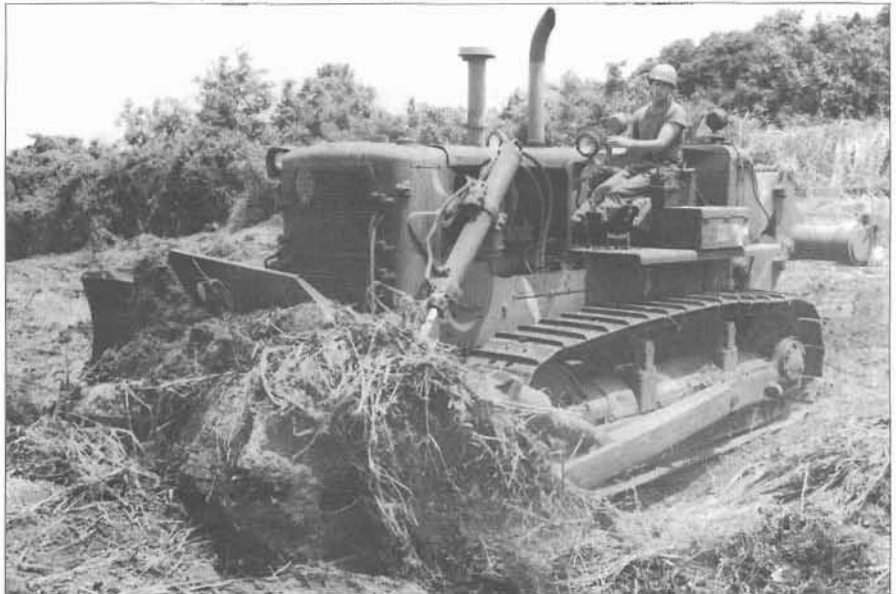
One of the task force's missions was to improve drainage in flood-prone areas. The task force used Guard and Reserve equipment.
