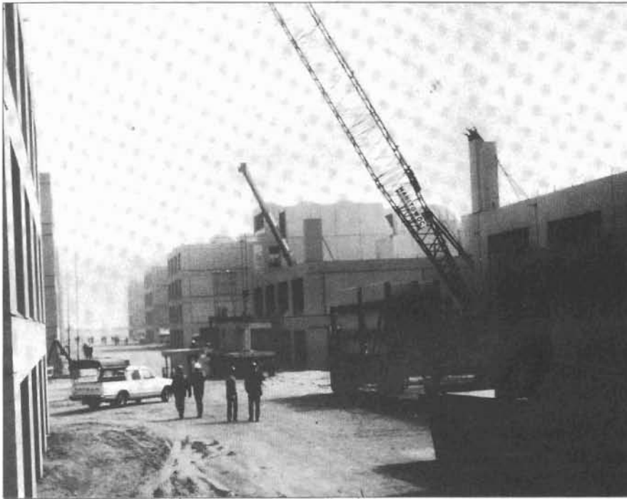
The $7 billion King Khalid Military City is the largest construction project ever handled by the Corps. It will be completed late this decade.
