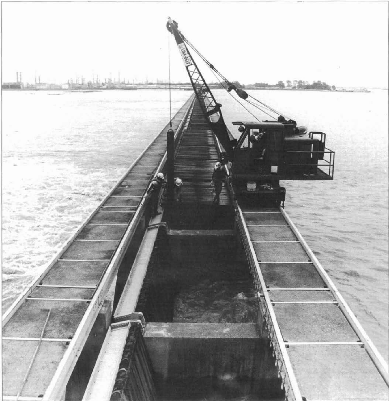
A crane atop Bonnet Carre spillway lifts one of the 7,000 "needles" to begin opening one of its bays. (U.S. Army photo.)
