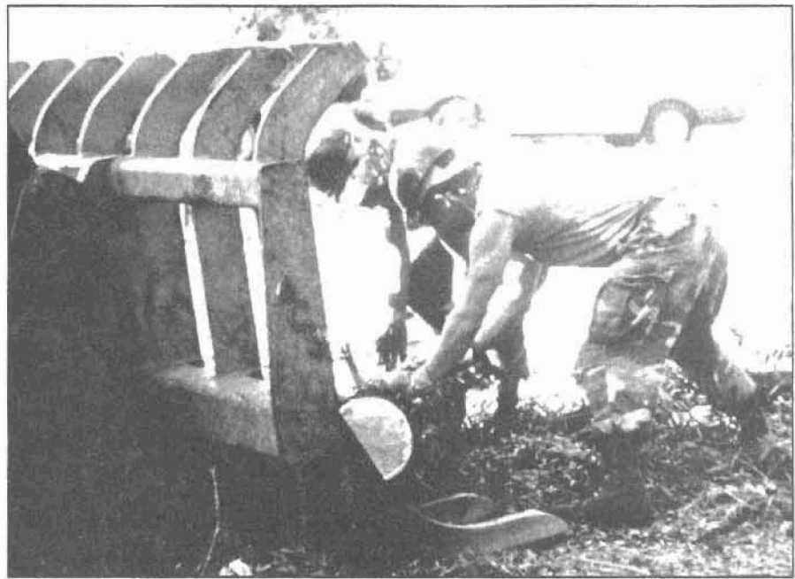
Members of the 202d Red Horse Engineer Squadron, as part of the joint relief effort, load a log onto an articulating front loader. (Photo by TSGT Rose Reynolds, USAF.)
