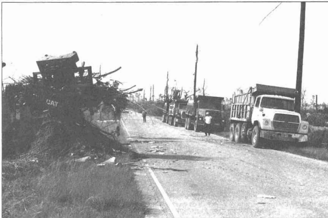
Military and civilian contracted engineer equipment hauls debris from public rights-of-way to dump sites.
