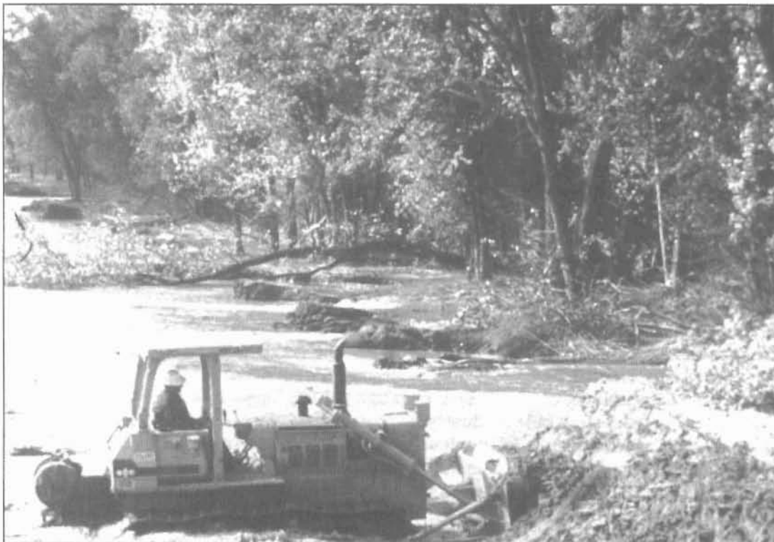
Photo this page: At Sny Island, Illinois, a dozer clears dredged material from the riverbank.
