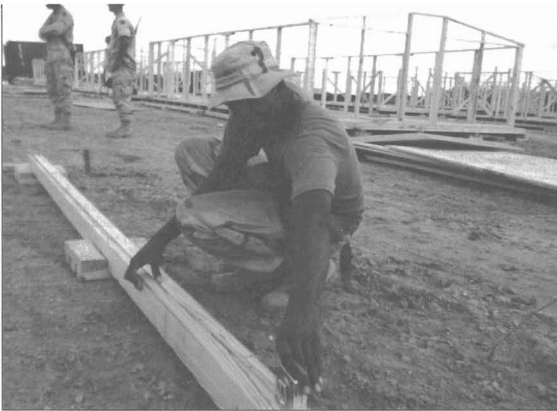
PV2 Mebane of 1st platoon, B Company, marks floor joist positions on a strongback tent beam.
