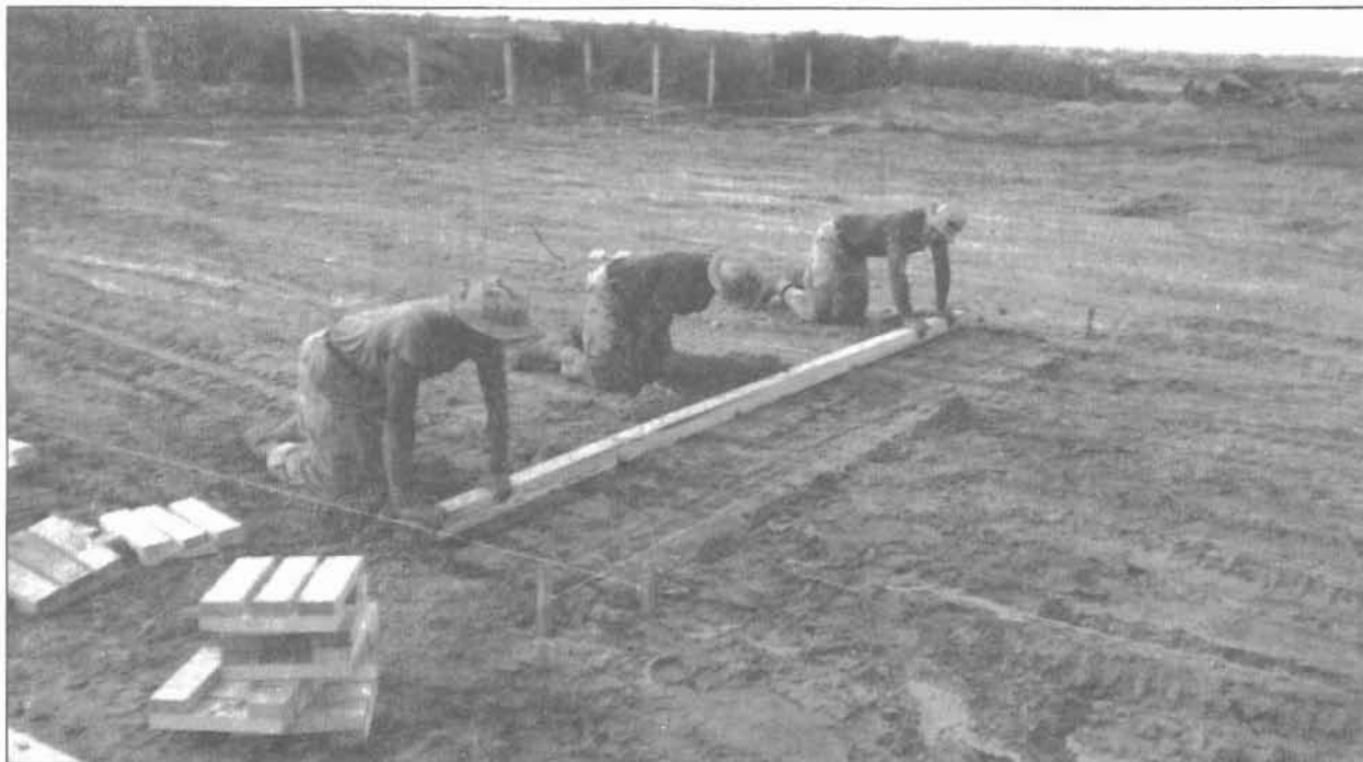
SPC Martin, SPC Fullwood and SPC Massey (left to right) of 1st platoon, B Company, level the ground prior to placing strongback footings.
