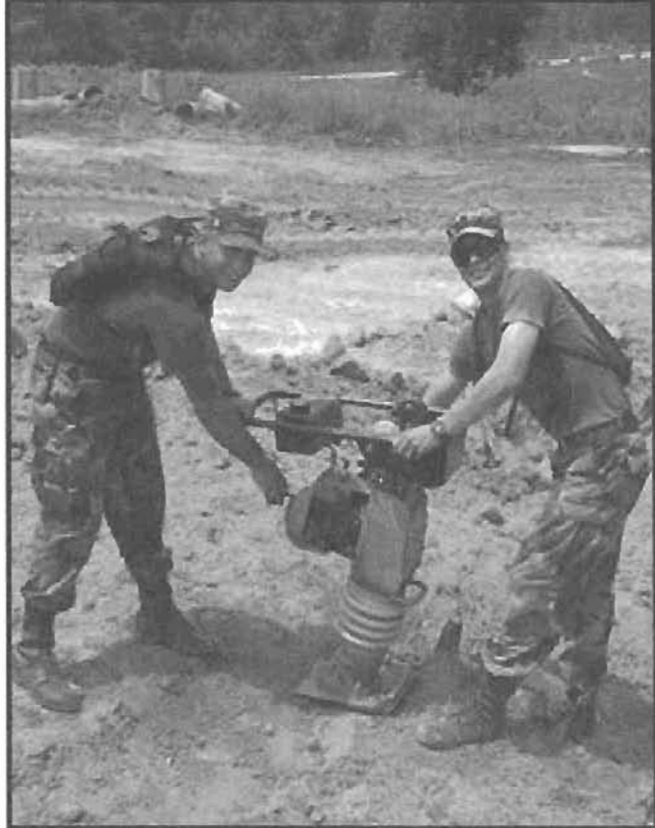
Soldiers from 1st Platoon use a hand tamper to compact soil on top of dual 18-inch plastic corrugated culverts.
