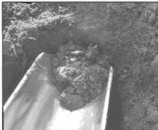
Radioactive contamination was discovered during earthwork.
