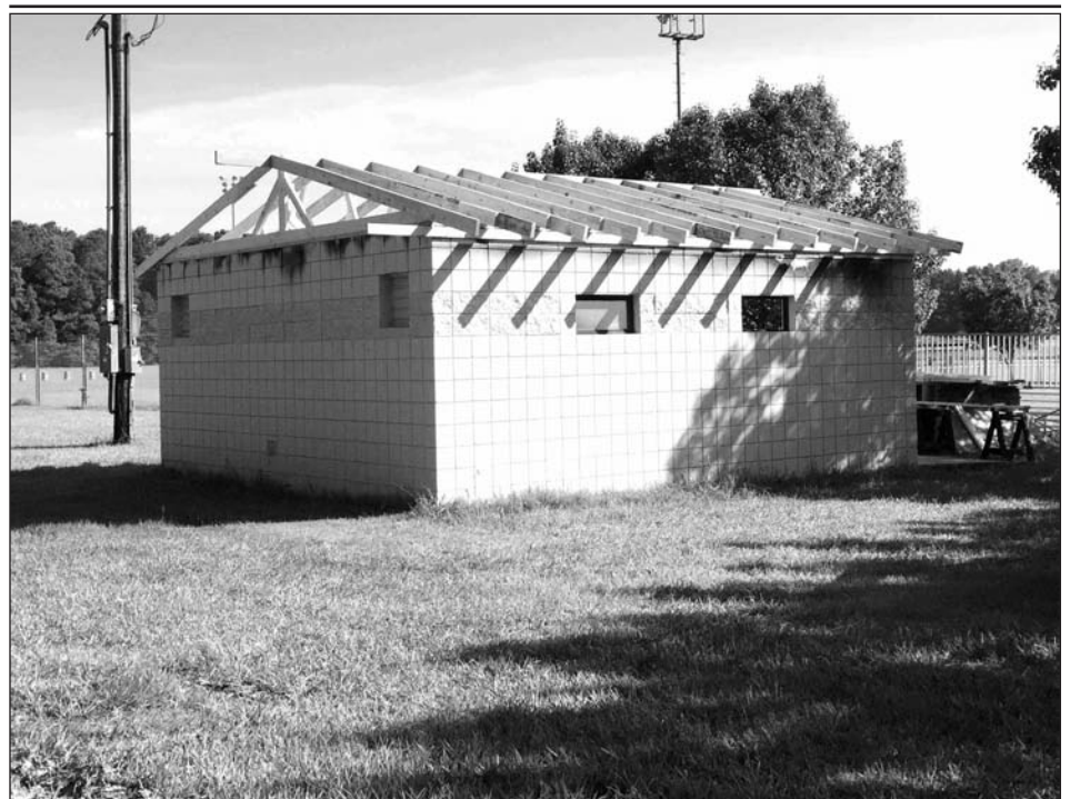
Pine Bluff Arsenal's Directorate of Public Works began reconstruction on a bathroom located on the installation's parade/ball fields. On March 10, the Arsenal's Fire Department, Directorate of Emergency Services, responded to a fire at the building. The fire was put out within minutes of arrival. The roof and men's side of the bathroom were heavily damaged even though the fire was contained to the attic space. It is believed that an electrical issue caused the fire, according to fire department reports. U.S. ARMY PHOTO BY RACHEL SELBY
