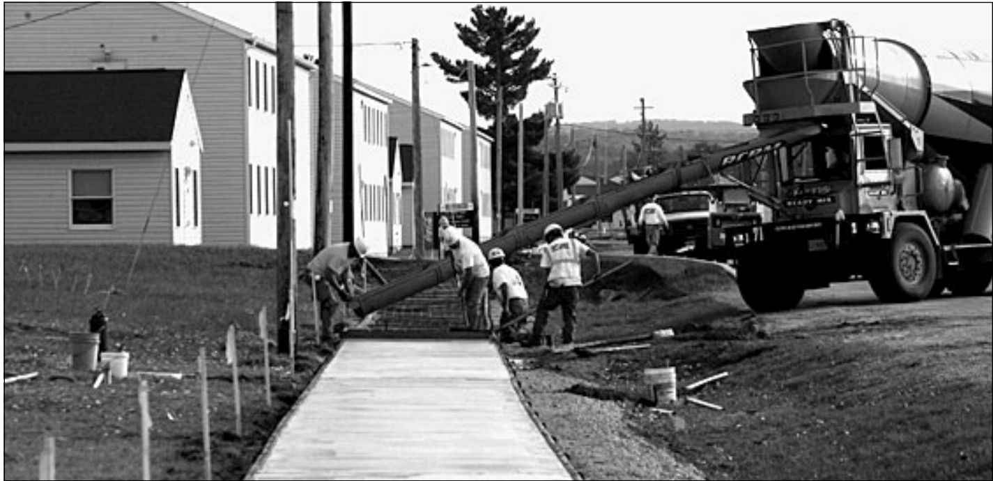
Contractors smooth freshly poured concrete as part of sidewalk construction at Fort McCoy.
