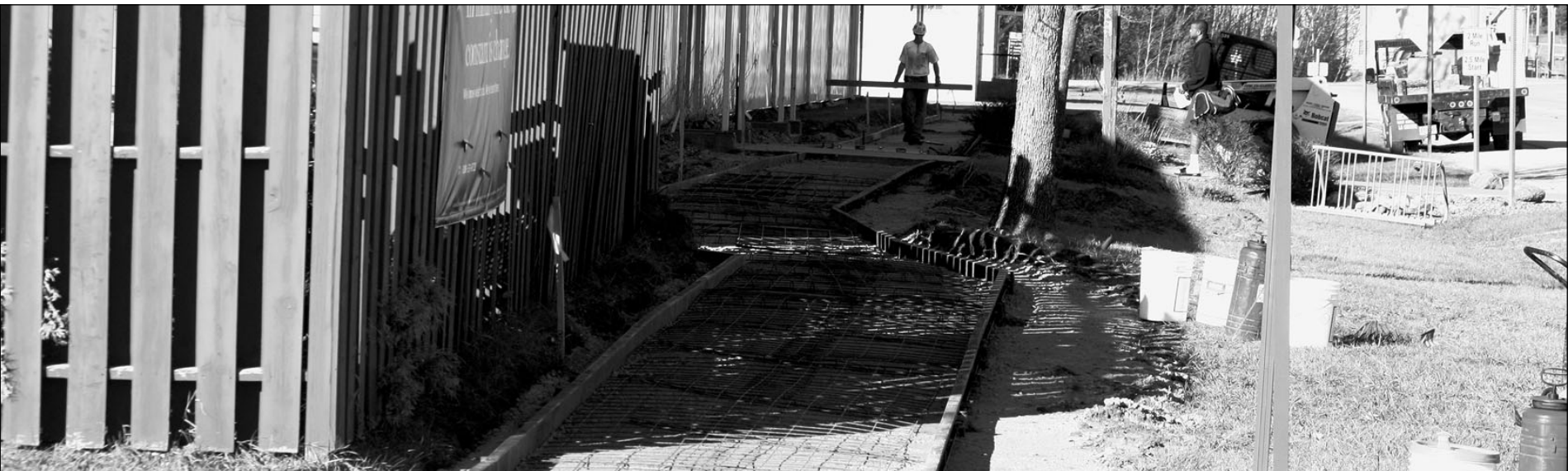
Contractors prepare a form for a new sidewalk in front of Rumpel Fitness Center.
