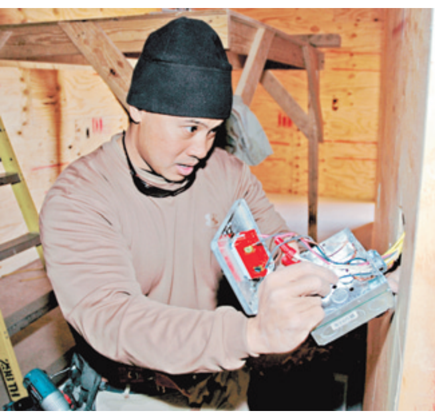
Spc. Dane R. Calvan, a 298th Engineer Detachment electrician from Kailua-Kona, Hawaii, installs a light switch at the newly built POL (Petroleum, Oil and Lubricant) Barn at Kandahar Airfield.
