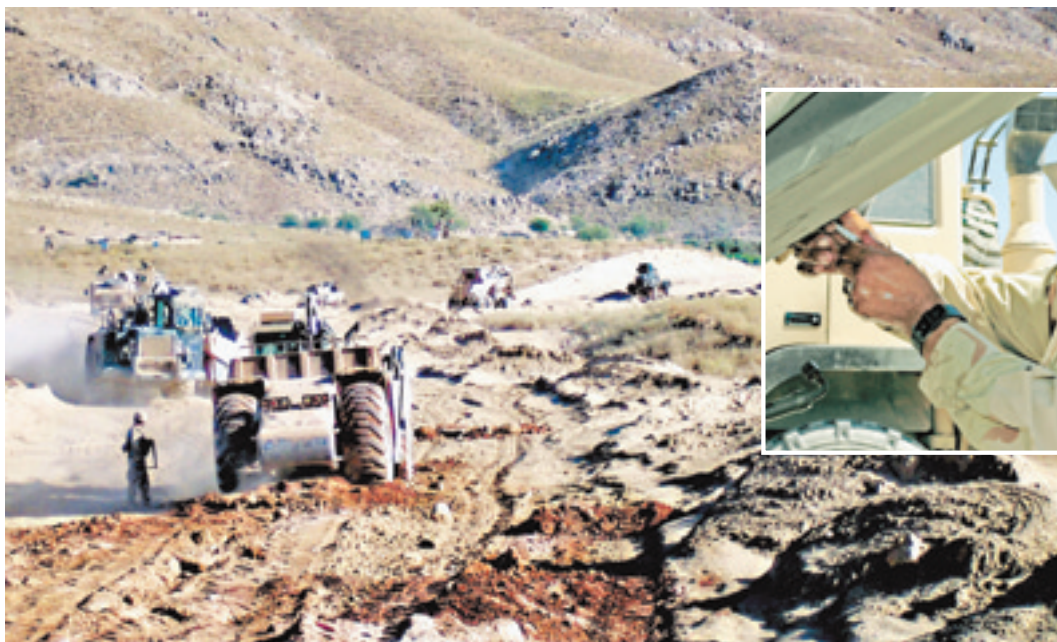
Task Force Pacemaker engineers crews cut path through a mountain pass to connect Tarin Kowt to Kandahar City, Aug. 26.
