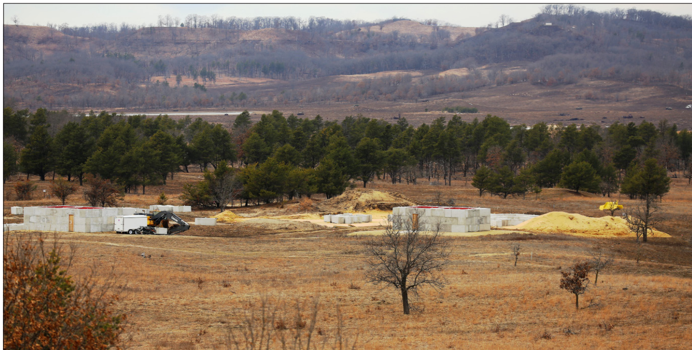
The construction area for the new Live-Fire Structured Collapse Venue Site is shown on Range 29 in late February.
