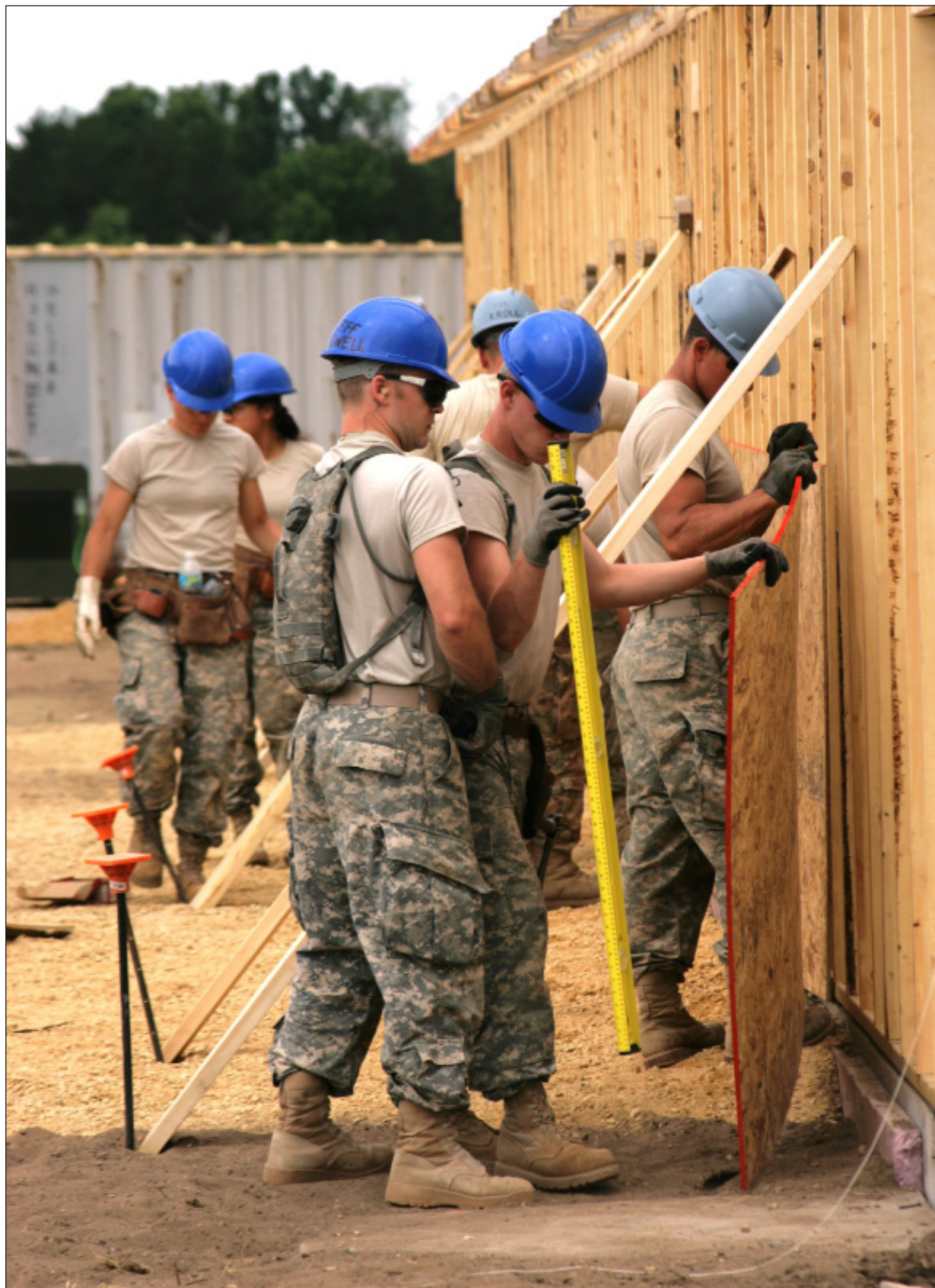
Soldiers with the Wisconsin National Guard’s 829th Engineer Company (Vertical) of Ashland and Spooner, Wis., work on a shower facility in June 2016 at Improved Tactical Training Base Freedom on Fort McCoy’s South Post.
