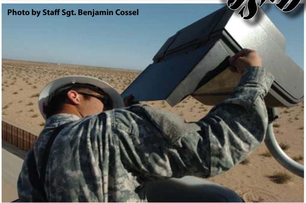
A Soldier with Task Force Diamondback works attaching covers to a high-density lighting pole in Yuma, Ariz.
