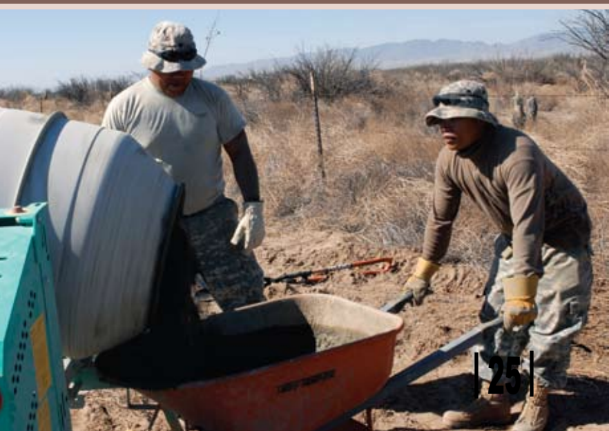
Soldiers from the Guam National Guard attached to Operation Jump Start-Arizona’s Task Force Diamondback pour concrete for fence posts during construction of a horse training academy enclosure.
