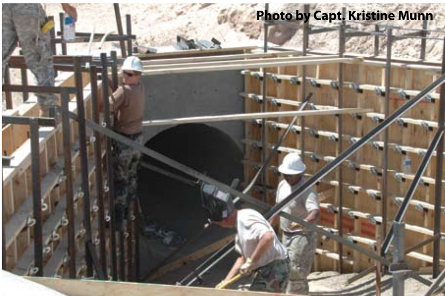
Soldiers of Task Force Diamondback work shoring up the security of a canal in Yuma, Ariz., that runs between the U.S. and Mexico.
