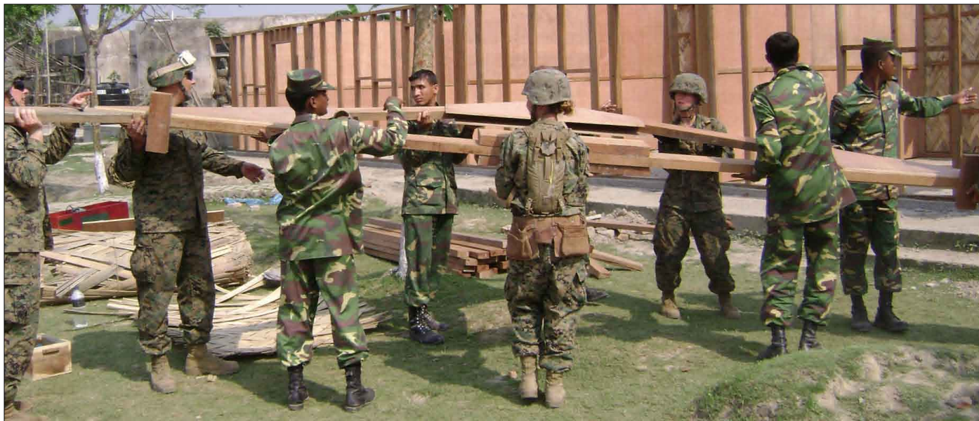
Marines of 1st Engineer Platoon, Bulk Fuel Company, 9th Engineer Support Battalion, 3rd Marine Logistics Group and Bangladesh Army soldiers of the 9th Engineer Battalion, 55th Infantry Division build a school in the town of Mongla March 14. The school was destroyed by November's Cyclone Sidr, which caused nearly 3,500 casualties and destroyed crops, homes, businesses and schools. Some estimates suggest a total of $450 million in damage. Photos courtesy of 9th ESB
