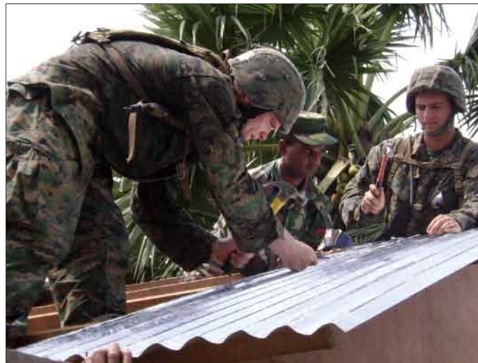
Pvt. Jesse Helsley (left), Bangladesh Army Sgt. Rahman Khalil and Cpl. Robert Knudson help put together the tin roofing for a new school house for an Islamic school in Mongla, Bangladesh March 22.
