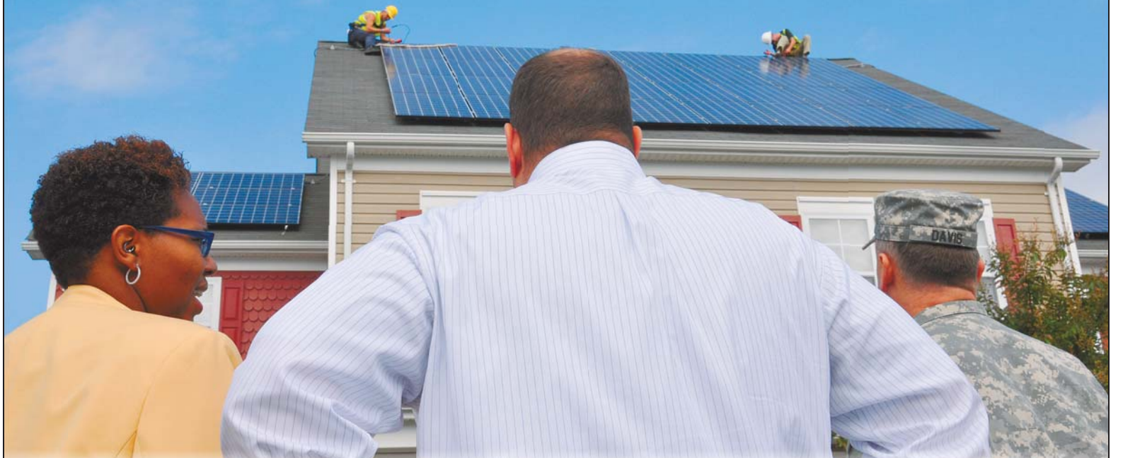
APG Garrison Commander Col. James E. Davis, right; Scott Kotwas, Corvias Military Living business director, center; and Keisha Brown, Corvias program development analyst, watch workers install solar panels on a Bayside Village home, Oct. 7. APG is the first Corvias installation to receive cost-saving solar panels through the Department of Defense Privatized Housing Solar Challenge initiative.
