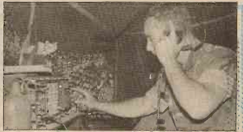
Sgt. Scott Saeger, switchboard operator, transfers calls from base camp to CSSD-37 on a SB3614 switchboard.
