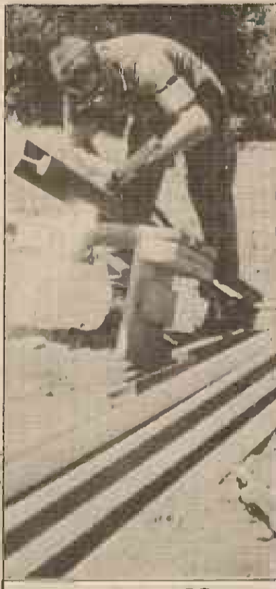
A welder from LSC, cuts lengths of steel girders while attached to CSSD-37.
