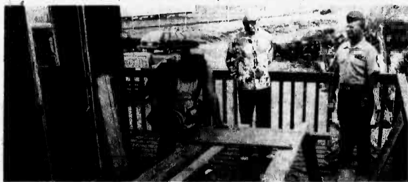
Retired Sergeant Major Bob Porter (c) and Station Sergeant Major Willie Trawick (r) check work being done by carpenter George Oshiro.
