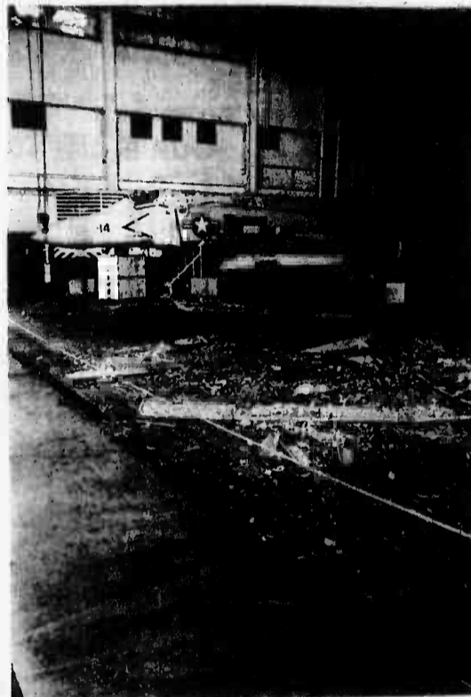
A portion of hangar 375's roof caved in during Hurricane Iwa. Home of Headquarters and Maintenance Squadron-24, Intermediate Level Maintenance Facility, a special shelter had to be erected to protect any further debris from hitting the aircraft.
