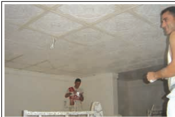
A new radio station construction site in Multaka, Iraq, is providing employment for local construction workers. This photo was taken August 20 during a coalition tour of the facility. (Photo submitted by Task Force 1-163 Infantry)
